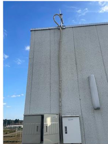
11ah antenna installed on the roof of the Tea Research Institute
